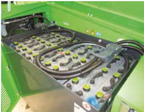
WATERING SYSTEM FOR BATTERY
